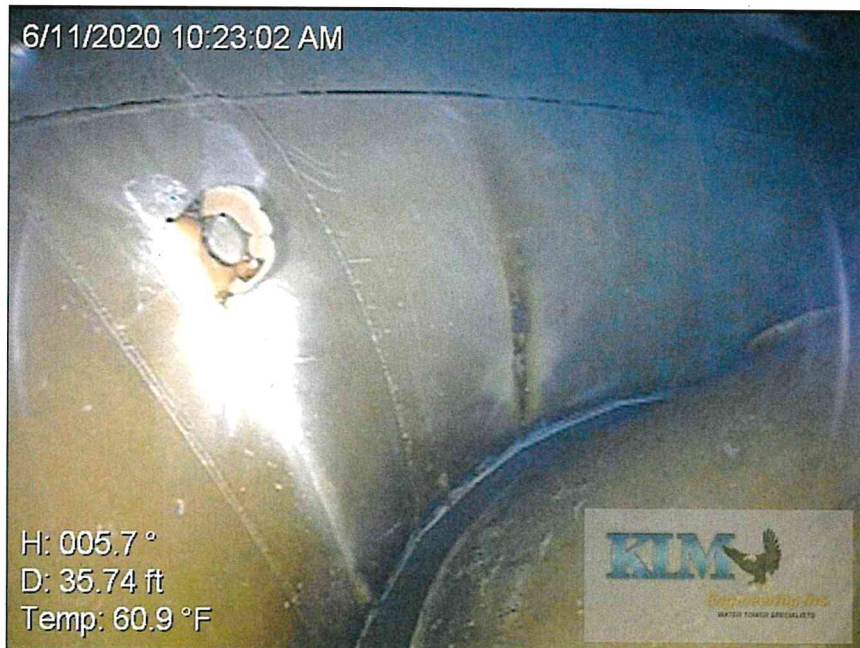
Photo No. 18 Condition of the bowl with a corroding rigging lug
