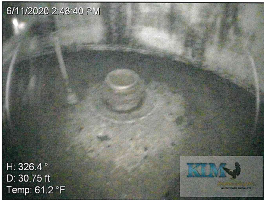
Photo No. 15 Condition of the floor with inlet pipe and cleanout plug with handle
