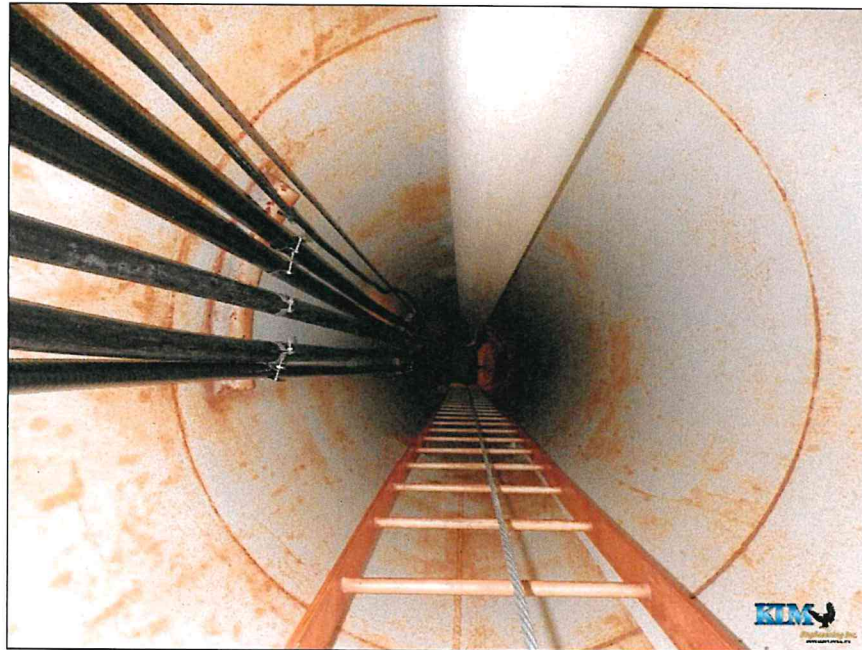
Photo No. 23 Condition of the drywell tube looking down with microcracking
