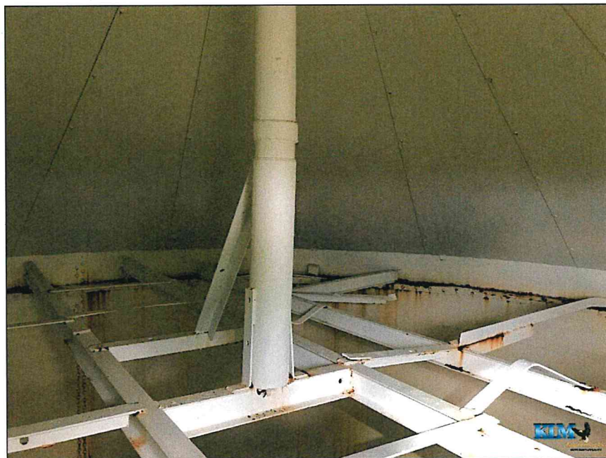
Photo No. 4 Condition of the roof plates and framing at the top of the shell
