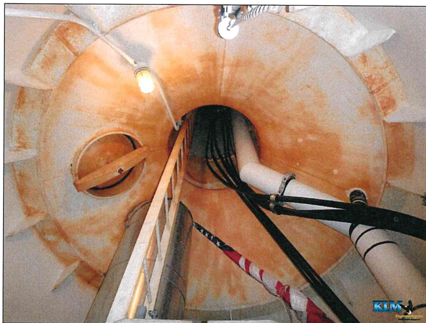
Photo No. 24 Overall condition of the bowl with microcracking
