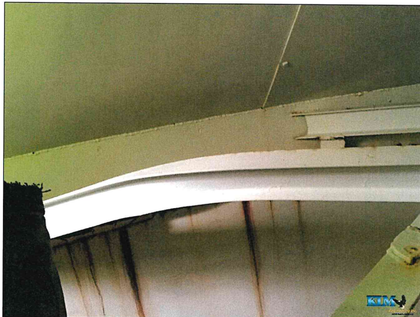
Photo No: 6 Condition of the roof to shell connection and bent top of shell framing
