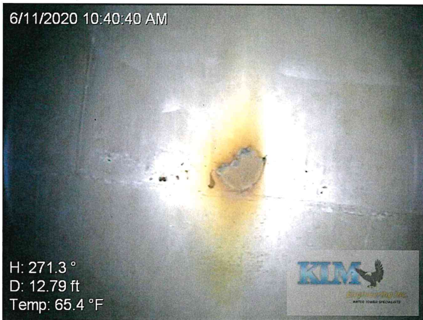
Photo No. 10 Condition of the shell with corrosion at a coating failure
