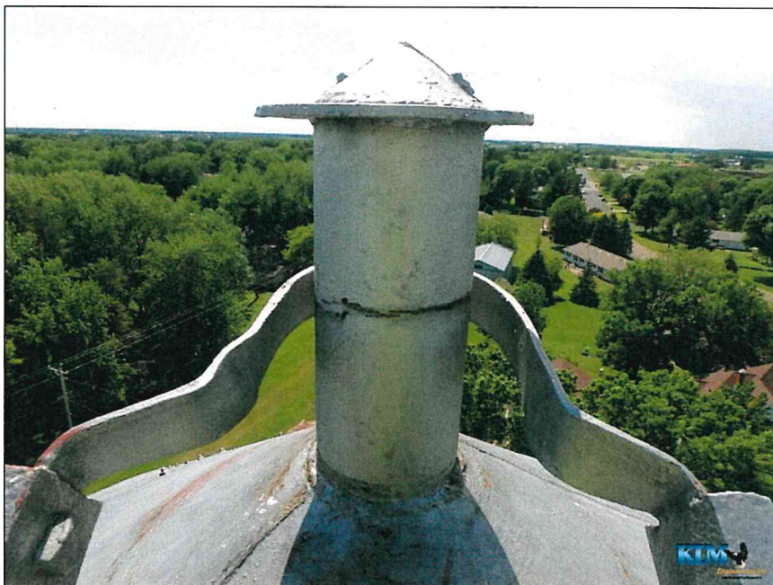
Photo No. 20 Top center ladder support, note there is no vent only the overflow pipe
