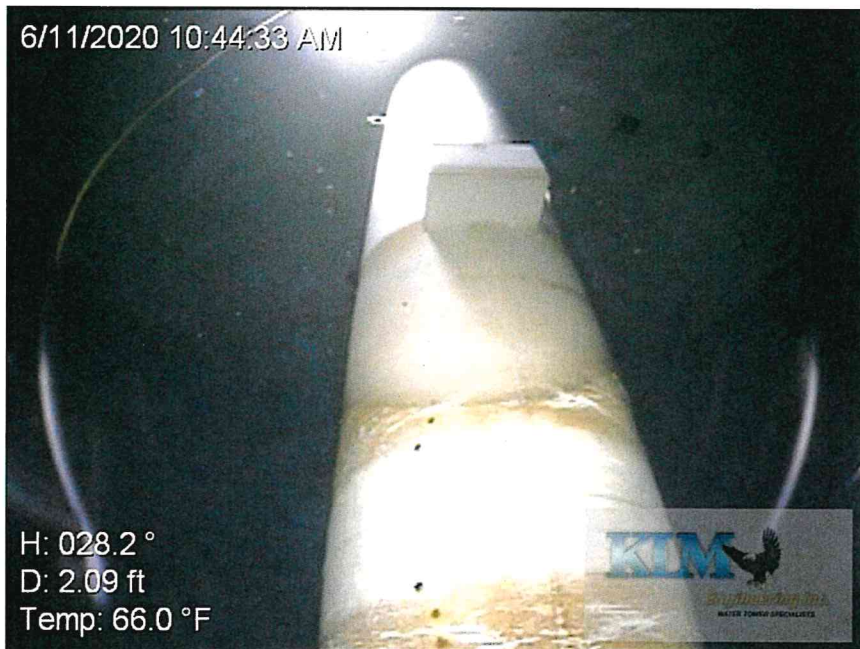
Photo No. 20 Drywell tube with corrosion nodules
