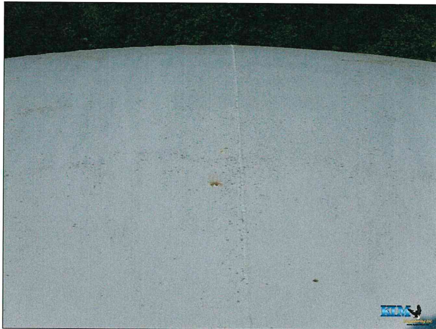
Photo No. 40 Condition of the roof with corrosion nodules and topcoat deterioration
