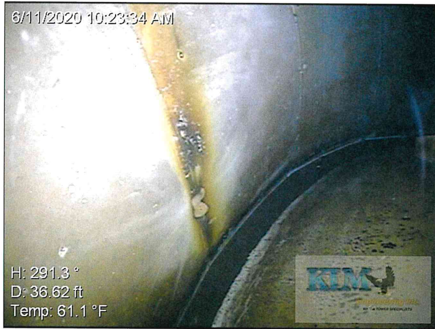
Photo No. 17 Corrosion in the bowl
