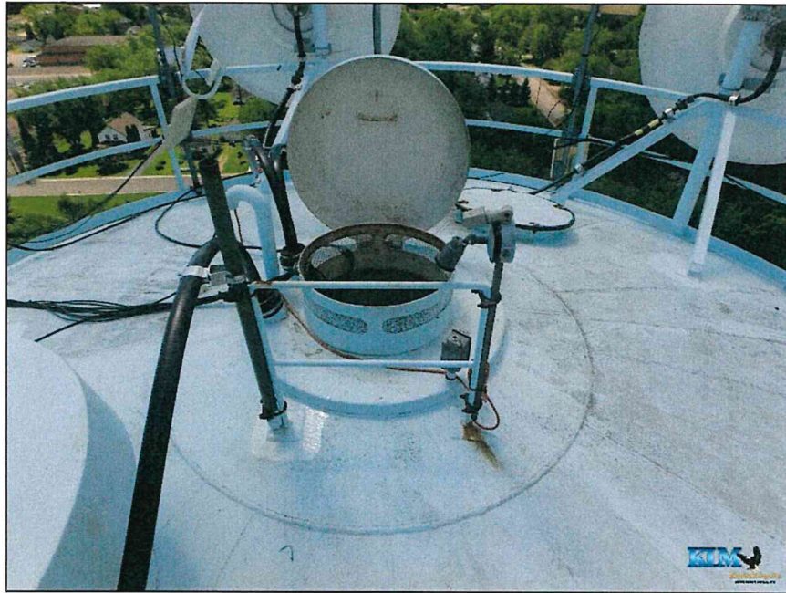
Photo No. 37 Condition of the top of the drywell tube
