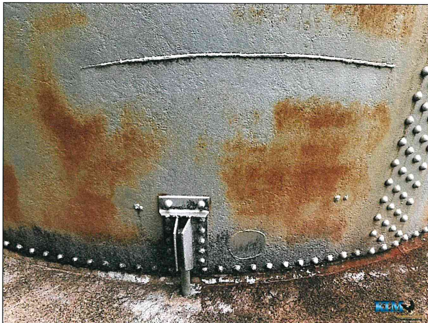
Photo No. 28 Condition at the base of the standpipe
