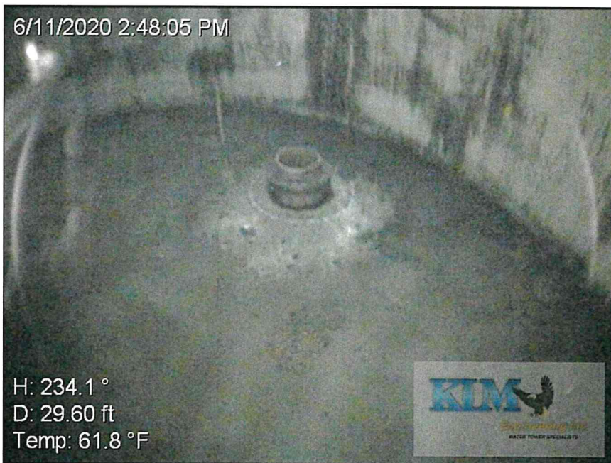
Photo No. 14 Overall condition of the lower shell course and bottom with inlet pipe
