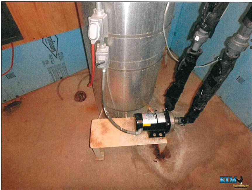
Photo No. 32 Inside the base cone inlet pipe enclosure with recirculation lines and pump
