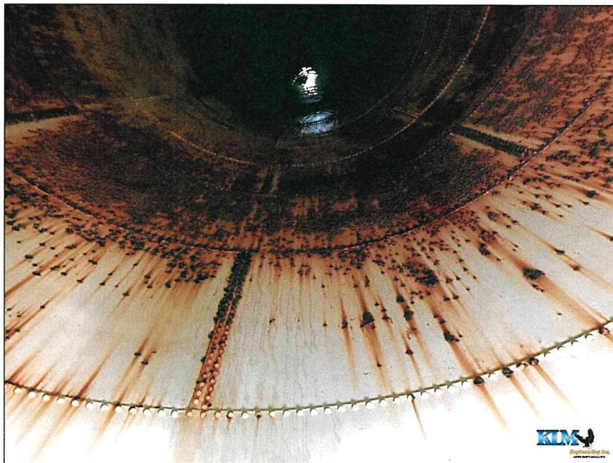
Photo No. 10 Shell corrosion
