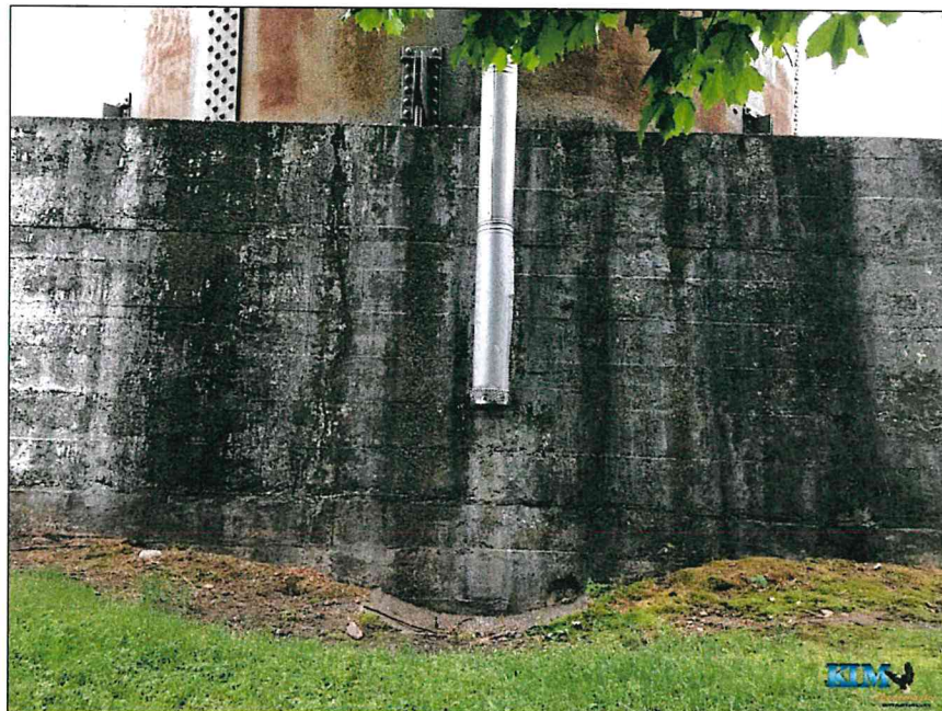
Photo No. 32 Condition of the base of the standpipe, concrete pedestal and overflow pipe
