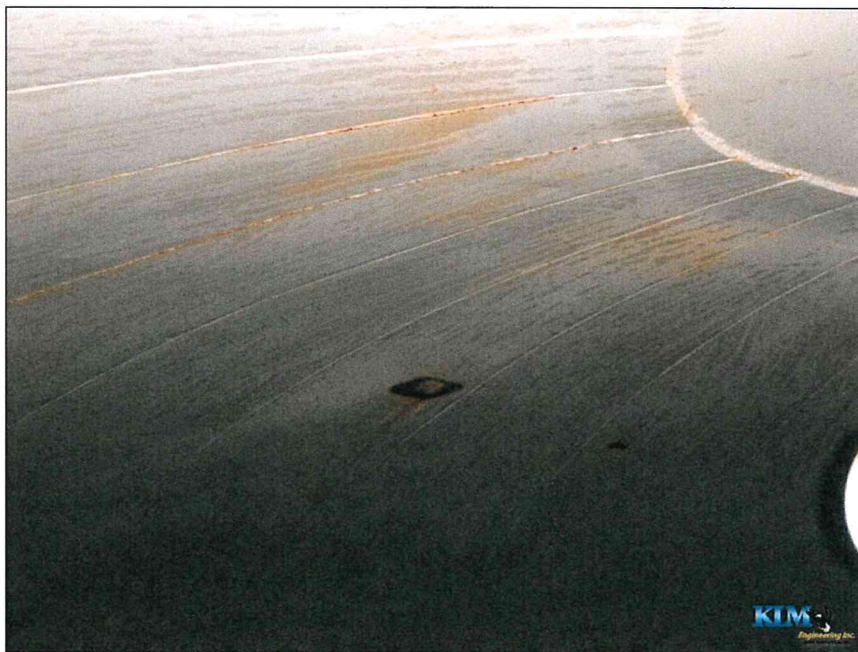
Photo No. 2 Overall condition of the roof with corrosion on plates and weld seams plus antenna installation burn marks
