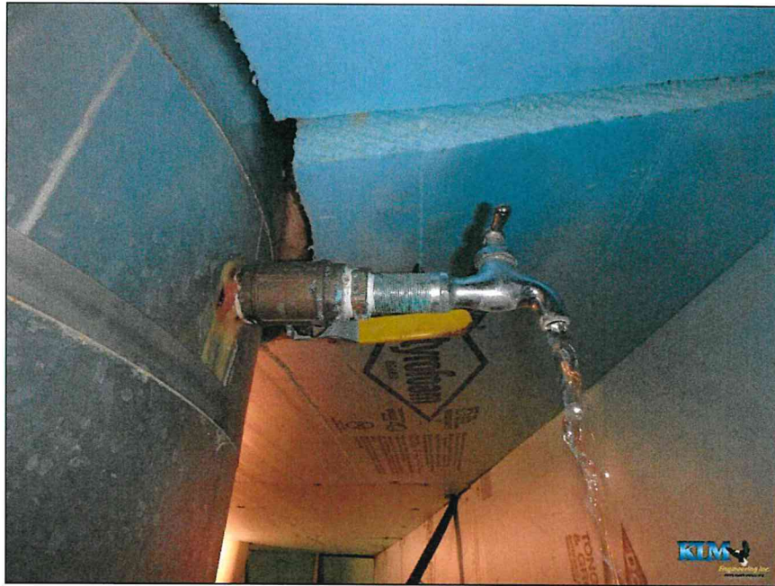
Photo No. 33 Sample tap on the inlet pipe in the enclosure
