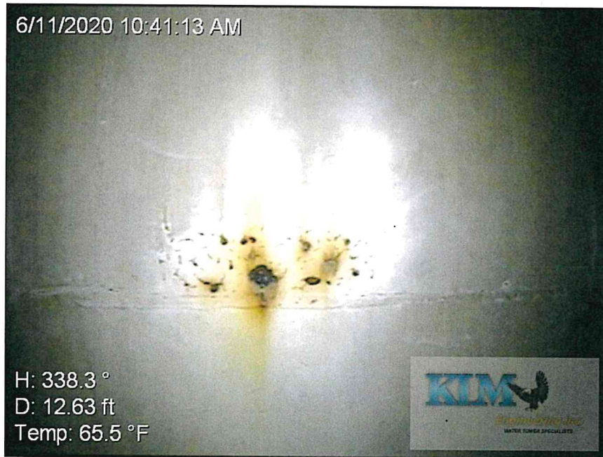
Photo No. 11 Coating failure on the shell
