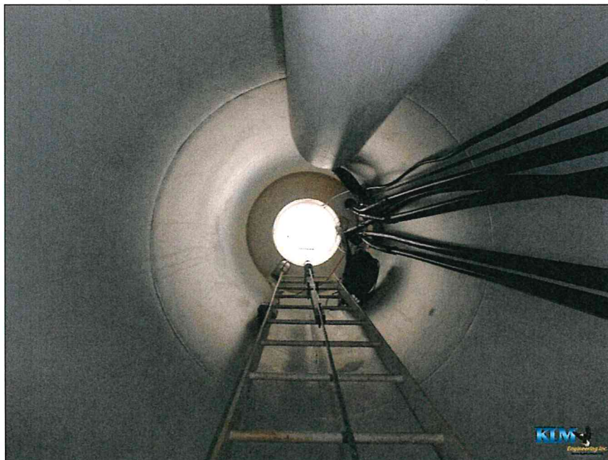
Photo No. 22 Top of the drywell tube looking up with coaxial cables and electrical conduit mounted to the access ladder in violation of OSHA
