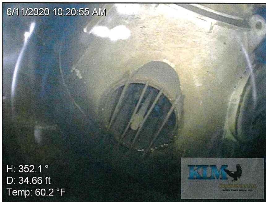
Photo No.16 Inlet pipe with recirculation line
