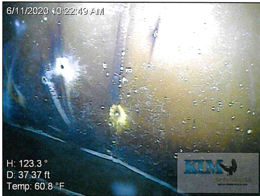
Photo No. 15 Corrosion in the bowl
