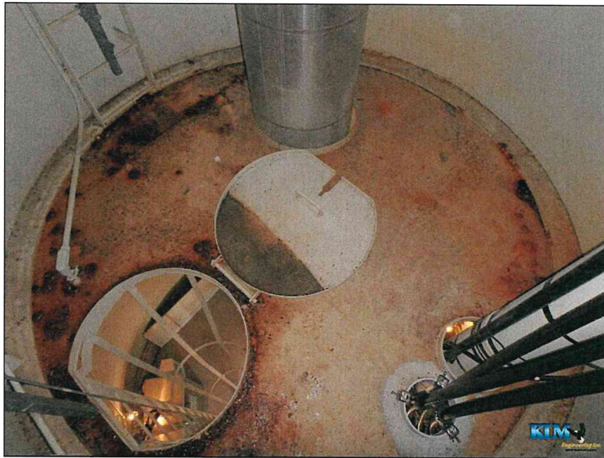
Photo No. 29 Condition of the lower condensate landing
