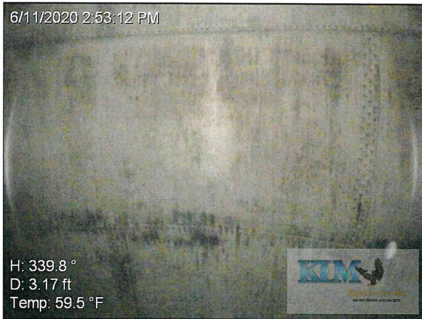
Photo No. 11 Lower shell condition below the current water line
