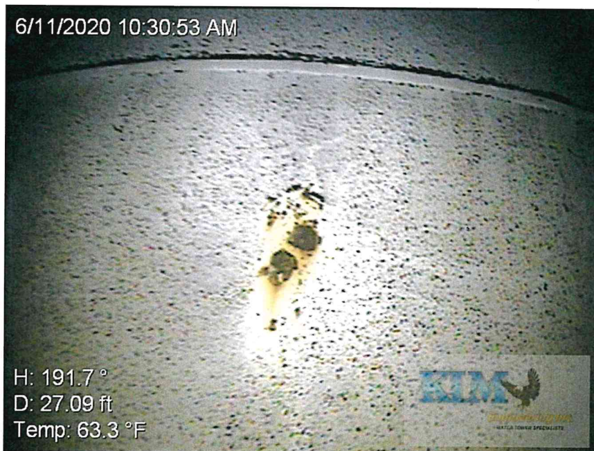
Photo No. 12 Coating failures in the upper bowl
