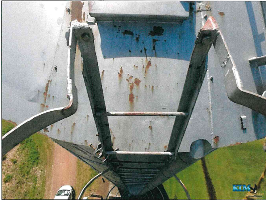
Photo No. 21 Condition of the roof at the top of the access ladder
