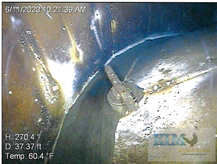
Photo No.14 Condition of the bowl with sediment, corrosion and cleanout coupling and plug
