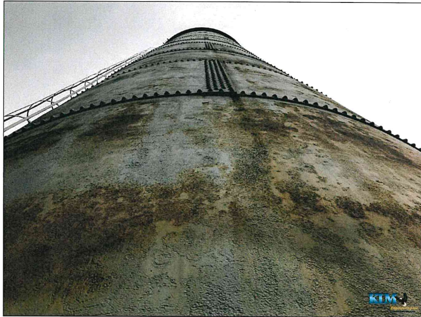
Photo No. 27 Condition of the lower shell courses with corrosion and pitting
