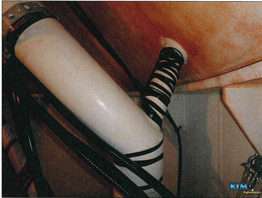
Photo No. 25 Condition of the bowl with cleanout pipe plumbed to the overflow pipe
