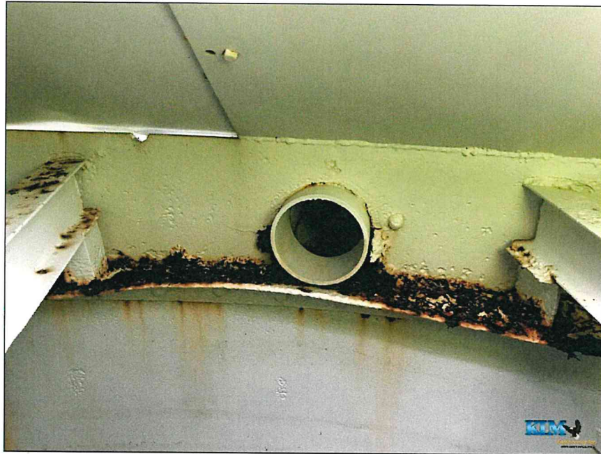
Photo No. 5 Condition of the lower roof with an unwelded roof panel, sill angle corrosion and the overflow pipe inlet
