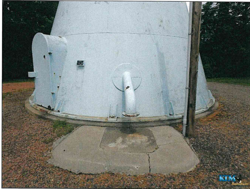
Photo No. 45 Condition of the base cone with overflow pipe discharge and splash pad
